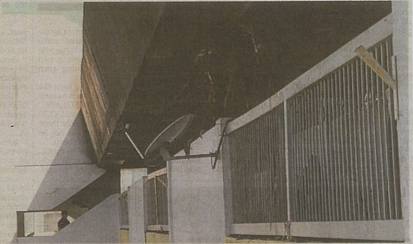
The aftermath: Initial findings found that the cause of the fire at Block 70 of the Sri Sabah flats in Cheras was not firecrackers but wiring issues, says Muhammad Salleh. — WILLIAM GARY/The Star
