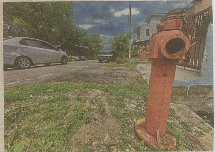
Not usable: A fire hydrant that has been vandalised. — FAIHAN GHANI/The Star
