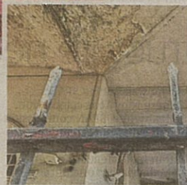
(Left) Bangunan Sultan Abdul Samad is still popular with tourists. (Inset) Badly damaged ceiling at BSAS, which is in need of repair and restoration.
