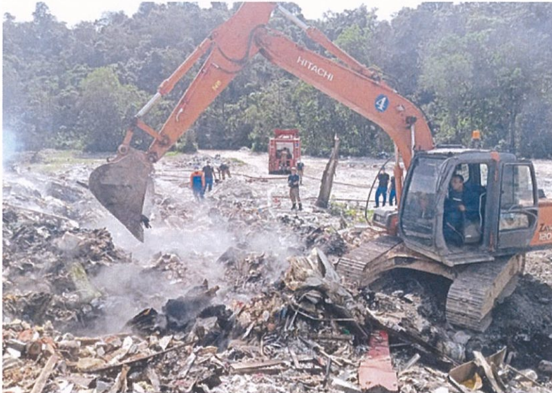
MBSJ Rapid Response Team and Seri Kembangan Fire and Rescue Department tending to the fire at an illegal dumpsite in Seri Kembangan.
