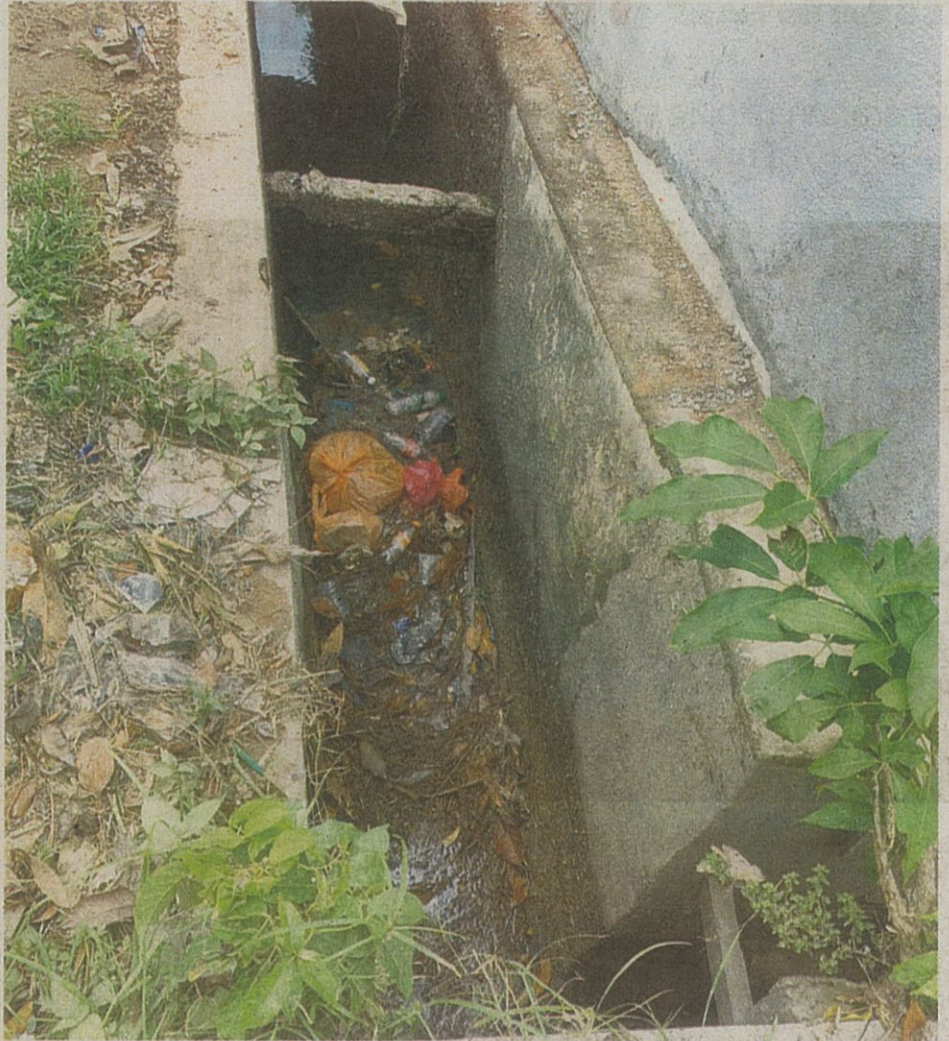
Limited frequency of inspections by the council has failed to address ongoing problems such as clogged drains, leaving the area prone to flash floods.
