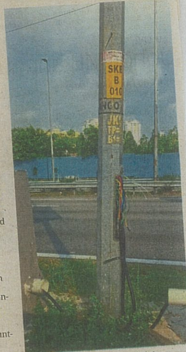
Exposed non-standard street lighting connection along the Federal Highway.
