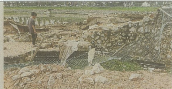
A boy walking on the collapsed water retention pond bund in Taman Seri Alam. — Filepic
