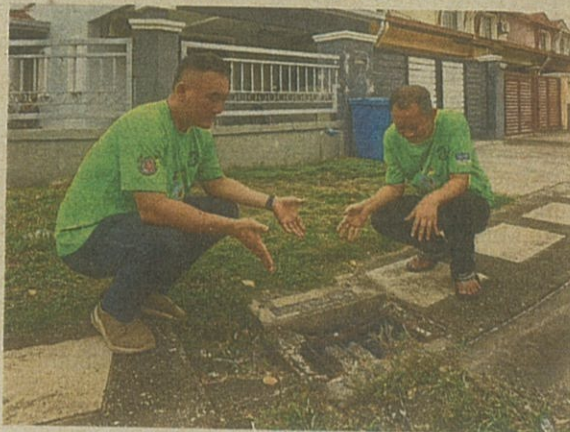
Siow (left) with Tan showing a broken drain cover in Jalan Setia Impian U13/4Q, Setia Alam. — SHAARI CHEMAT/The Star
