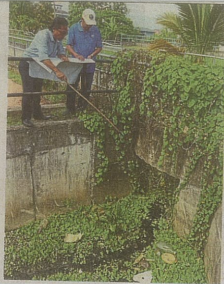
Mohd Rayme (left) with contractor Zamsari Sani checking on a heavily silted monsoon drain and its outlet along Lorong Seri Banang 14A/KS02. — KK SHAM/The Star
