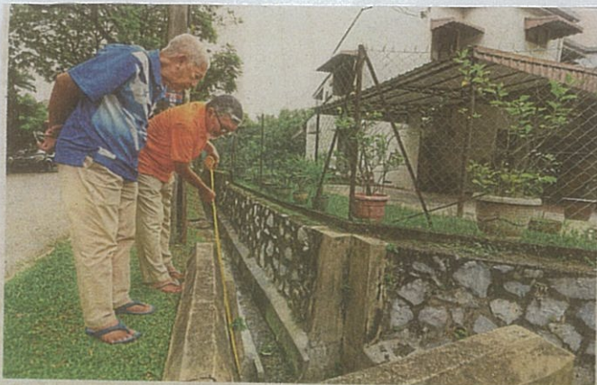
Azusaini (right) discussing the flash flood issue with resident Ahmad Nazli, while checking the depth of the sump. — Photo: CHAN TAK KONG/The Star
