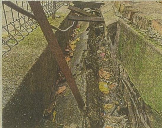
The wall of a drain behind a food court in Persiaran Mergastua in Kepong, Kuala Lumpur has collapsed, impeding the flow of water.
