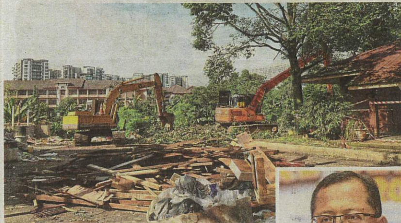
MBPJ brings in excavators to clear debris and stabilise the riverbank of Sungai Kayu Ara beside the Lembah Subang PPR. (Inset) Mohamad Zahri says MBPJ offered help in the interest of public safety. — ART CHEN/The Star
