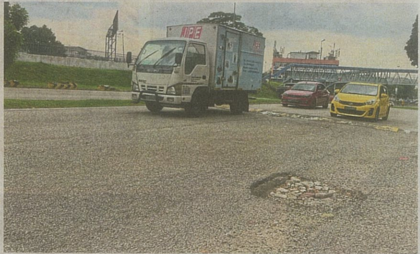
A pothole on Jalan Belimbing, near the entrance to Taman Bukit Belimbing in Balakong.
