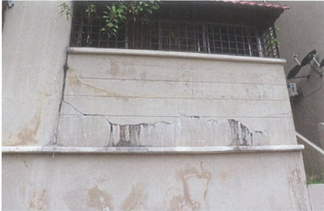
Dallas Villa Pandan Heights JMB says lack of maintenance funds, because of defaulters among owners, has delayed repairs such as for these walls. — Photos: LEW GUAN XI/The Star
