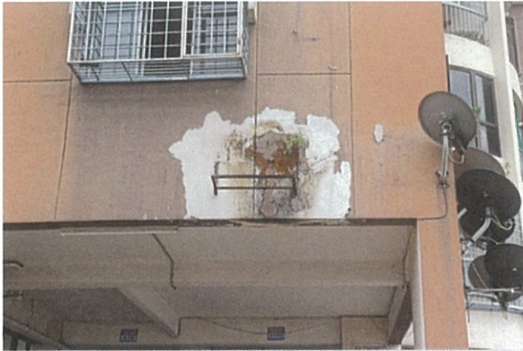
Dallas Villa Pandan Heights JMB says lack of maintenance funds, because of defaulters among owners, has delayed repairs such as for these walls. — Photos: LEW GUAN XI/The Star
