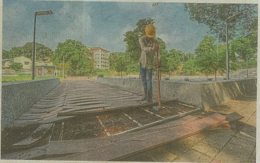
Warped decking planks being removed at Dataran Klang@Padang Chetty that is undergoing repairs and upgrading work. — IZZRAFIQ ALIAS/The Star
