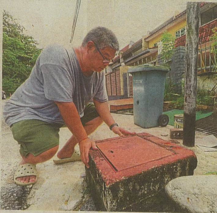
Lee keeps an eye out for defective fire hydrants in Taman Desa. This chamber hydrant can easily be overlooked due to the missing H pillar. — SAMUEL ONG/The Star
