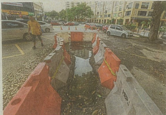
A pothole in the middle of Jalan PJU 8/2 in Damansara Perdana, Petaling Jaya, has turned into a dangerous one-metre obstruction.
