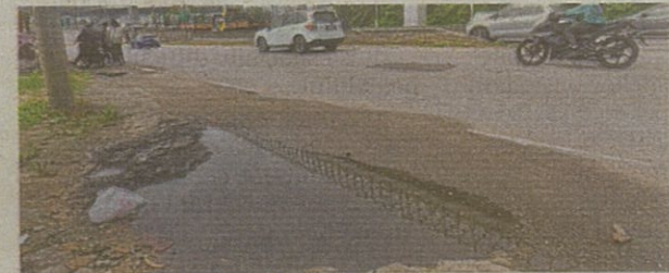
Stagnant water on the uneven roadside. — RAJA FAISAL HISHAN/The Star
