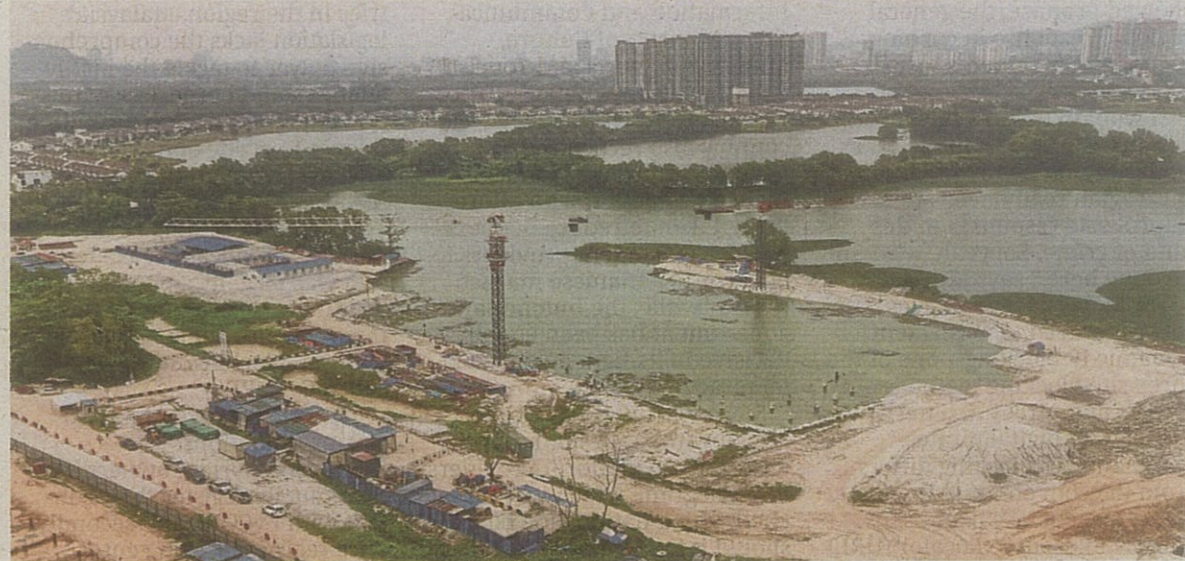
Murky cause: An aerial view of the embankment collapse at the Sungai Rasau water intake point in Taman Mas, Puchong. — SHAARI CHEMAT/The Star
