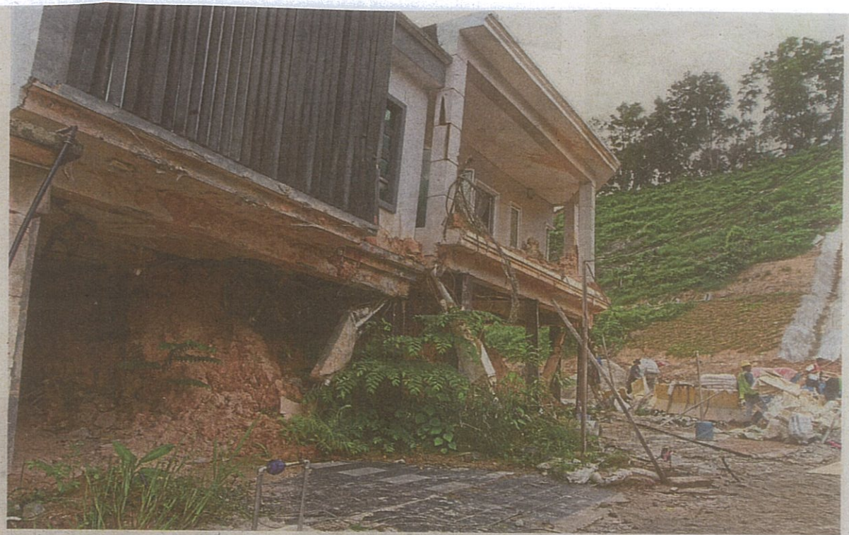
Broken drainage contributed to the Taman Bukit Permai landslide in 2022. — Filepic
