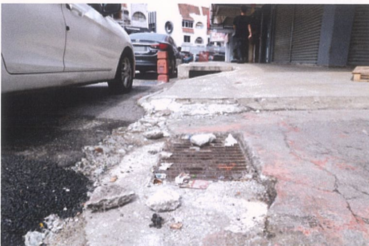
Uneven roads and pavements endanger pedestrians.
