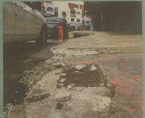
Uneven roads and pavements endanger pedestrians.
