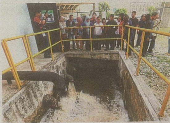
Maimunah and Tan during a working visit to the pump house at Jalan Chan Sow Lin, Kuala Lumpur. — LOW BOON TAT/The Star
