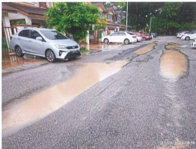
Lorries using residential roads have caused visible damage, with potholes becoming more apparent during the rainy season.
