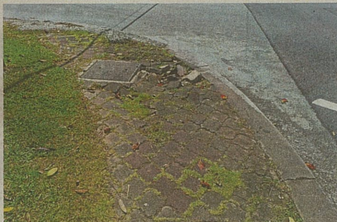
Pavement defects along Jalan Gasing and throughout Petaling Jaya make walking dangerous.
