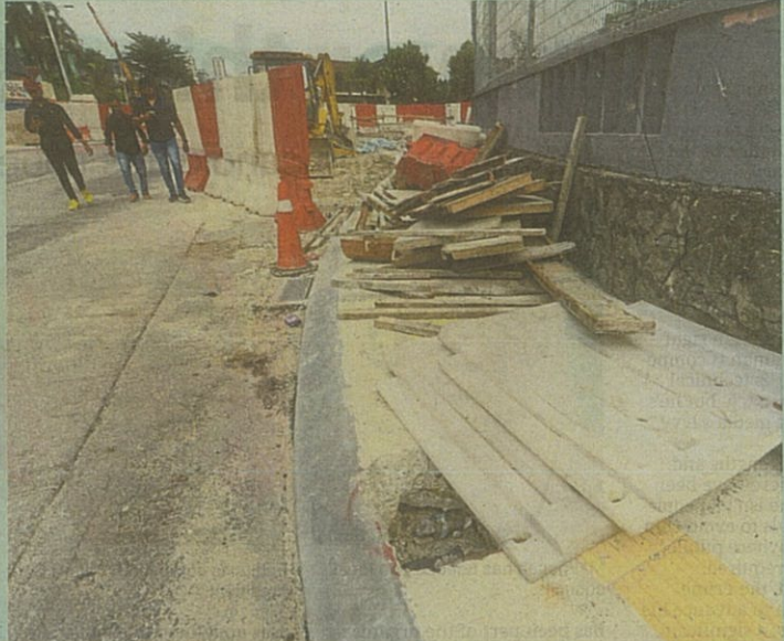
Contractors should never leave construction debris on walkways. — Filepic
