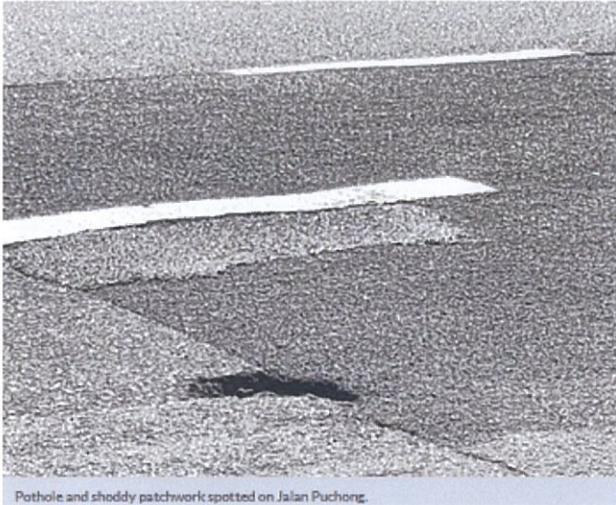
Pothole and shoddy patchwork spotted on Jalan Puchong.
