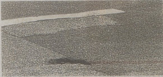
Pothole and shoddy patchwork spotted on Jalan Puchong.
