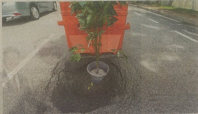
Many road users have suffered vehicle damage, bodily injuries, and some have even lost their lives due to long-unrepaired potholes and road iron covers that sit lower than the road surface. — THE SUN
