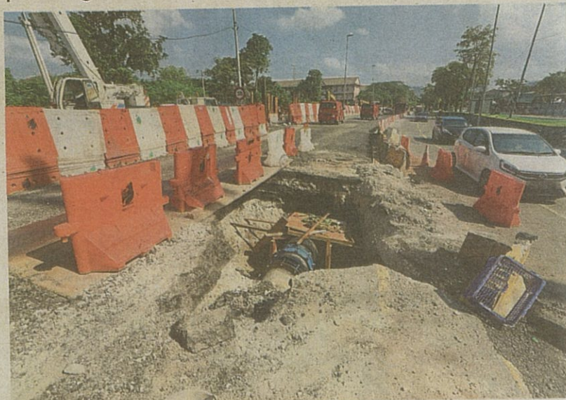
The sinkhole is caused by a burst pipe. To fix the sinkhole, a pipe with special modification is needed for repairs, says DBKL. — LOW LAY PHON/The Star
