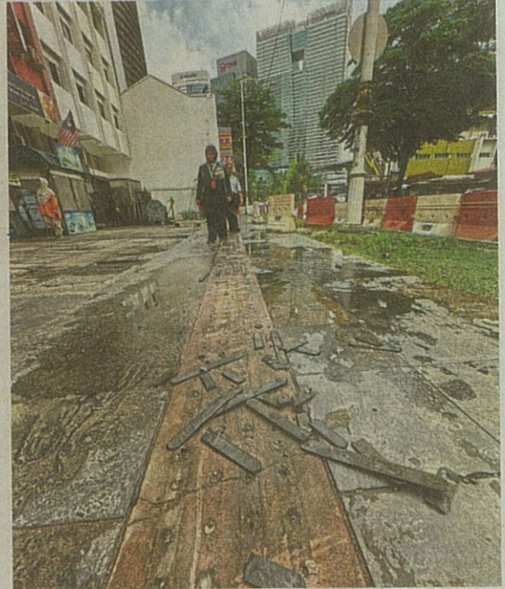
Visually-impaired pedestrians wading along a damaged tactile path in Brickfields, Kuala Lumpur. — Photos: LOW LAY PHON/The Star
