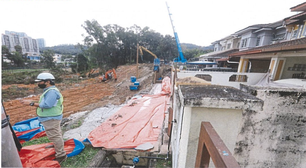
A total of 29 residents were evacuated from nine houses following the landslide in Taman Wawasan Puchong. — Filepic
