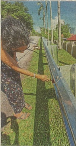
Carmel showing a wobbly reflector on the recently installed guardrail along Jalan Tinggi 6/12 in Petaling Jaya.
