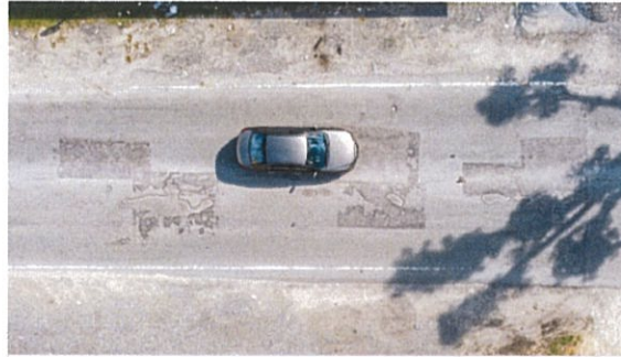
The poor condition of Jalan TK4/5 in Taman Kinrara.
