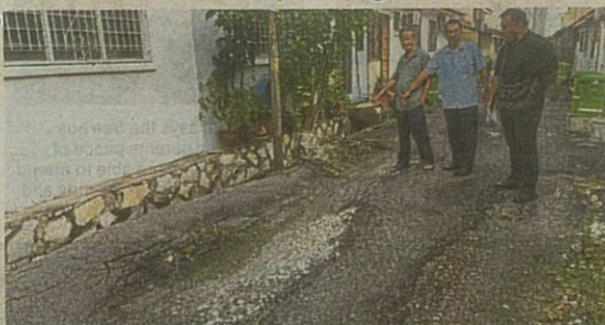
(From left) Tan, Yee and Zulhelmi highlighting part of the damaged stretch of the back lane between Jalan Lang Putih 7 and Jalan Lang Putih 8 in Kepong Baru Tambahan.
