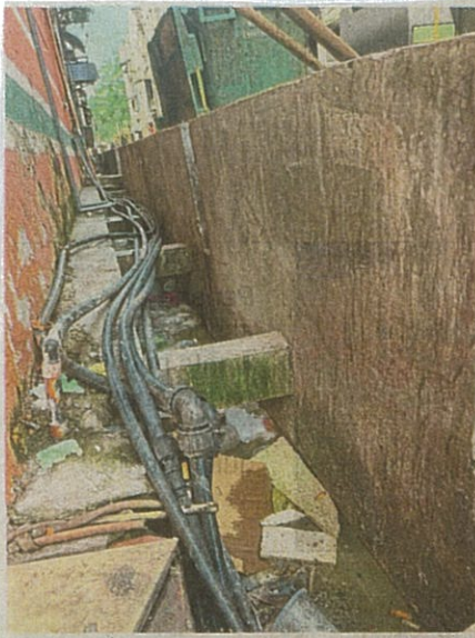
Illegally installed water pipes snaking in drains in Jalan Khoo Teik Ee, Kuala Lumpur, hamper cleaning efforts.
