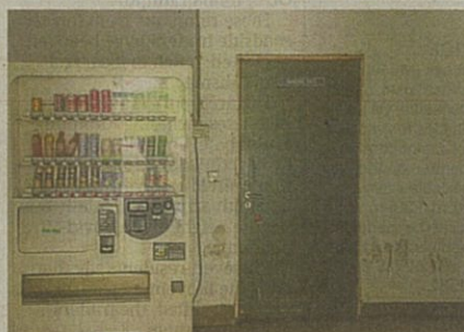
A vending machine hindering wheelchair-users' access to the toilet in Kompleks Tun Sambanthan, Brickfields. The toilet door and signage don't meet the requirements.
