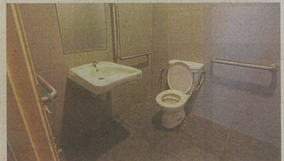
This toilet at the DBKL-owned Kompleks Tun Sambanthan is not built to specification as the hand rails and toilet bowl are too close, making it a challenge to manoeuvre a wheelchair.
