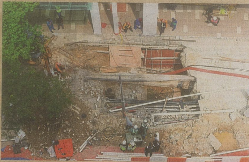
Aerial view of workers at the sinkhole in Jalan Masjid India, Kuala Lumpur. An Indian tourist fell into the 8m hole on Aug 23 and her body has not been recovered. — Photos: Filepic
