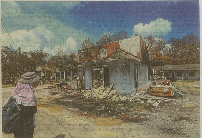
Inspecting the aftermath: A woman taking a closer look at a damaged structure in Kampung Kuala Sungai Baru, Subang Jaya. — IZZRAFIQ ALIAS/The Star
