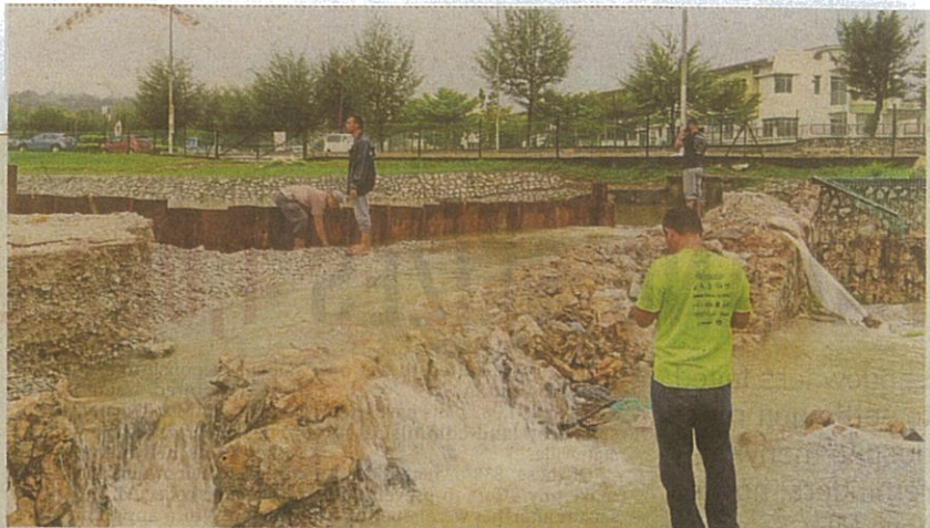
Water flowing through a damaged barrier at the Taman Seri Alam retention pond in Sungai Buloh yesterday. NSTP PIC BY FAIZ ANUAR
