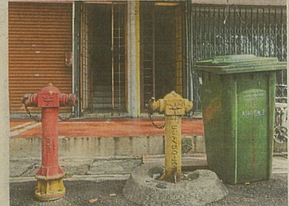
Above: Based on 2024 data, Kuala Lumpur has 18,424 fire hydrants, comprising 12,280 public hydrants (red) and 6,144 private hydrants (yellow).
