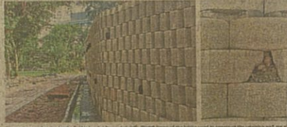
The retaining wall at the Astaka field is believed to be leaning slightly. Slipped some of the bricks used to construct the retaining wall are of
