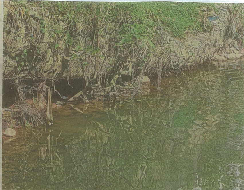
Damaged riverbank along Sungai Kuyoh near the National Hockey Stadium in Bukit Jalil, Kuala Lumpur. — Courtesy photo
