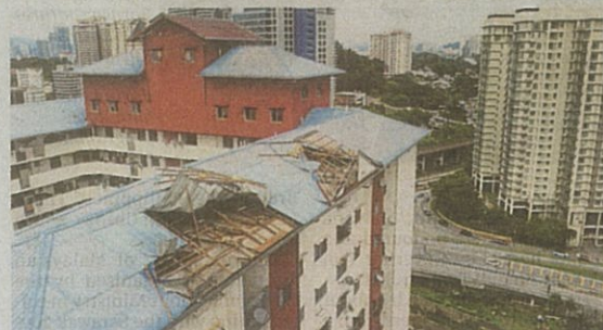
The roofs of Apartment Putra Ria Bangsar were blown off by unusually strong winds on Saturday.
