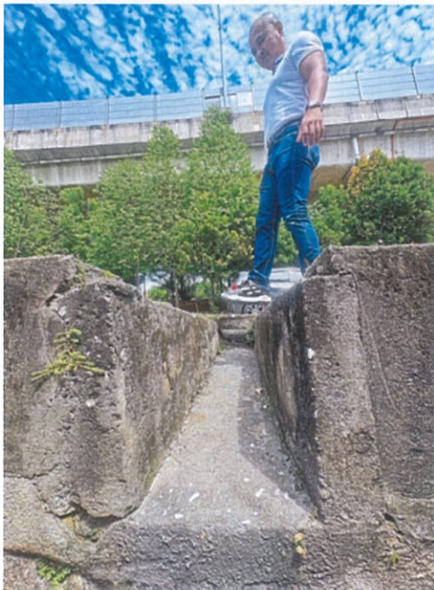
Goh says there have been reports of pedestrians and cyclists using the damaged pavement along Jalan SS12/4 in Subang Jaya tripping and falling into the drain. — Photos: MUHAMAD SHAHRIL ROSLI/ The Star
