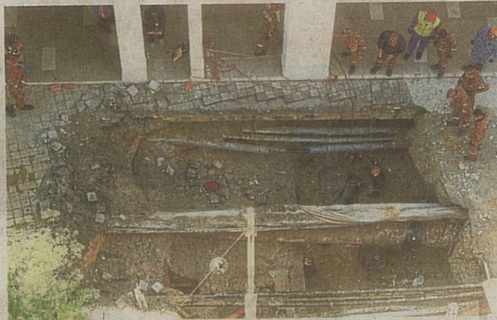
Search and rescue efforts are ongoing for Vijayalaksmi who fell into this sinkhole in Jalan Masjid India. — Filepic
