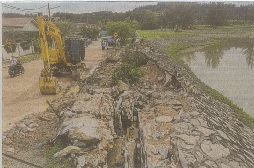
The collapsed water retention pond bund in Taman Seri Alam, Saujana Utama, Sungai Buloh, yesterday. BERNAMA PIC
