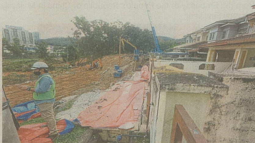
The 2023 Puchong landslide triggered by monsoon drain failure displaced residents from nine houses along Jalan Wawasan 3/9.
