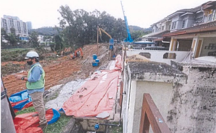
The 2023 Puchong landslide triggered by monsoon drain failure displaced residents from nine houses along Jalan Wawasan 3/9.
