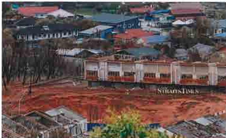
The Subang Jaya City Council had previously received one complaint regarding excavation works around the Putra Heights gas pipeline explosion site. NSTP/ALZUDDIN SAAD
